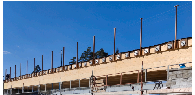
Fig. 9. Side view of the bridge at stage 1. The vertical flat bars and steel plates for the railings are present on the bridge.
