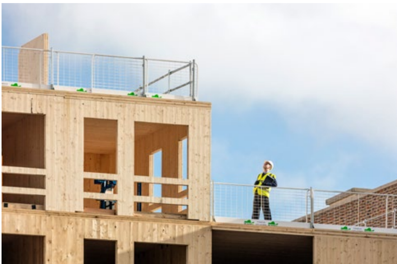
CLT external walls with pre-formed fall protection and window openings, Dalston Works
