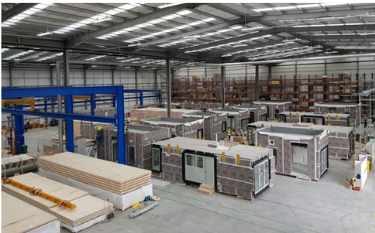
Volumetric modular factory showing the timber based units being finished with external membranes and windows
